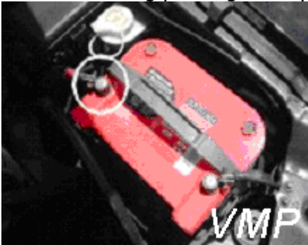
Wire orange wire to + battery side
